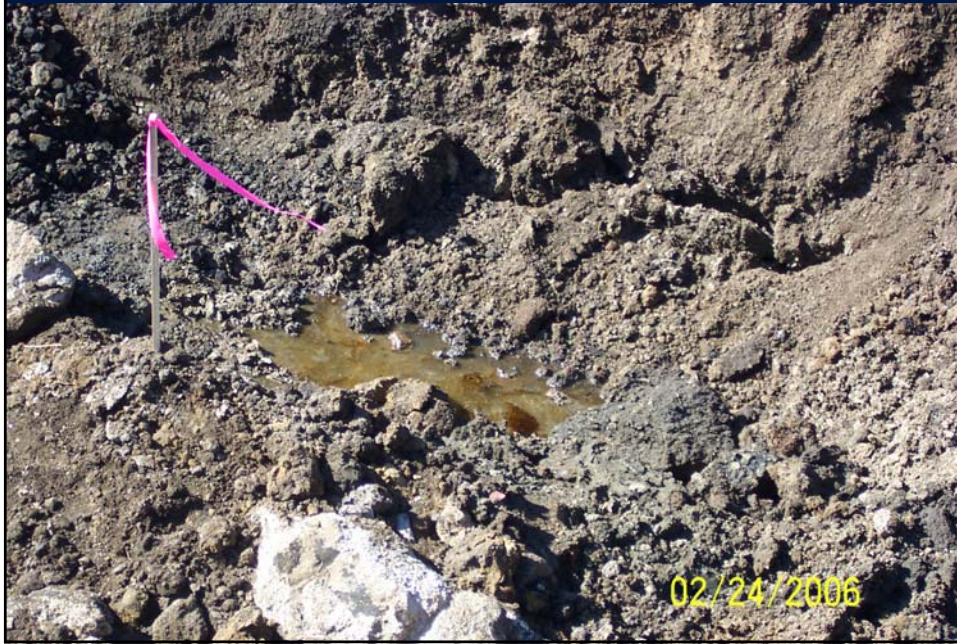
Underground Petroleum product oozing out of pipes with lead contamination
