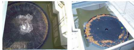
Saco's excess flow treatment systems at work.
